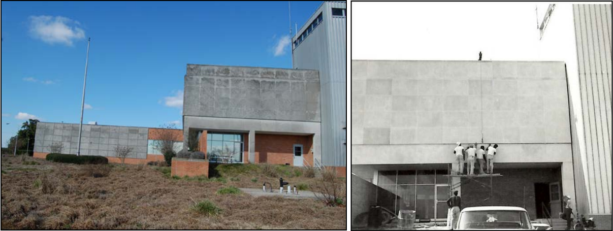
Figure 18. South side elevation of transmitter building, at left, and similar view of May 31, 1962, showing replacement of storm-damaged facing stone (both Site A) (source: VOA progress photographs file)
