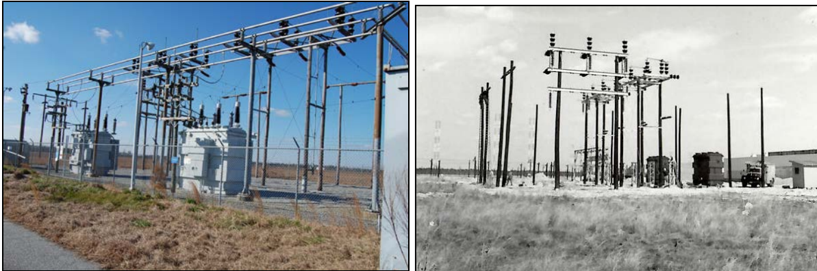
Figure 38. Electrical power transformers, insulators, bus bars, lines, and other components at outdoor power substation, at left; substation construction, April 16, 1962 (both Site A)
