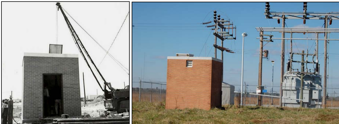
Figure 36. Installing well pumphouse 1, May 15, 1962 (source: VOA progress photographs file), at left; well pumphouse 1 and power substation, at right (both Site A)
