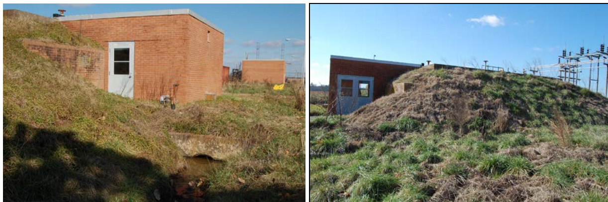
Figure 39. At left, looking northeast (from left to right) at brick retaining wall of reservoir, water storage building, and generator building; at right, looking west at generator building and reservoir set in man-made bank (both Site A)
