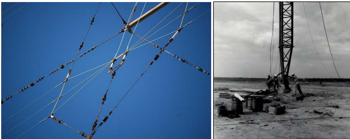
Figure 51. Multi-wire, bowtie-like dipoles suspended between towers at curtain antenna A-02, at left; curtain antenna A-07 being set on base plate, September 13, 1961, at right (both Site A) (source: VOA progress photographs file)
