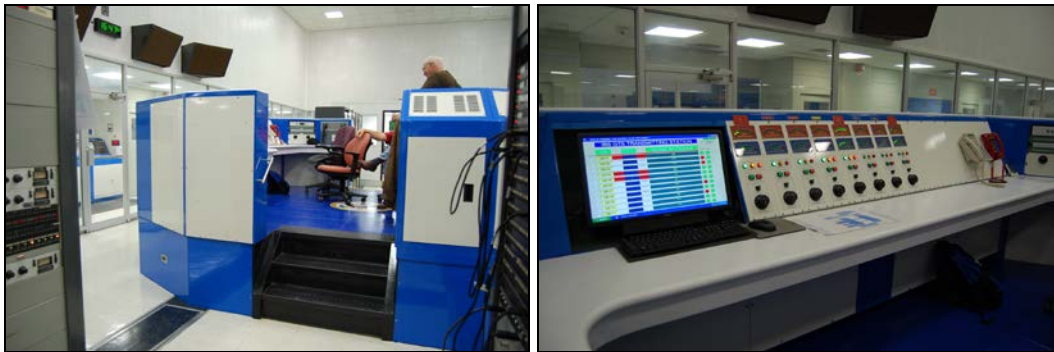
Figure 27. At left, looking east past switching equipment to control dais; at right, main console beyond which is the north transmitter hall (both Site B)
