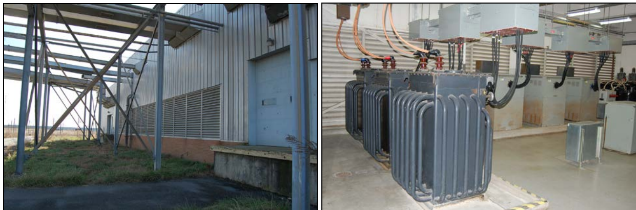
Figure 31. East rear elevation of transmitter building with ground-level louvers (Site A), at left, that ventilate the power distribution room (Site B), at right
