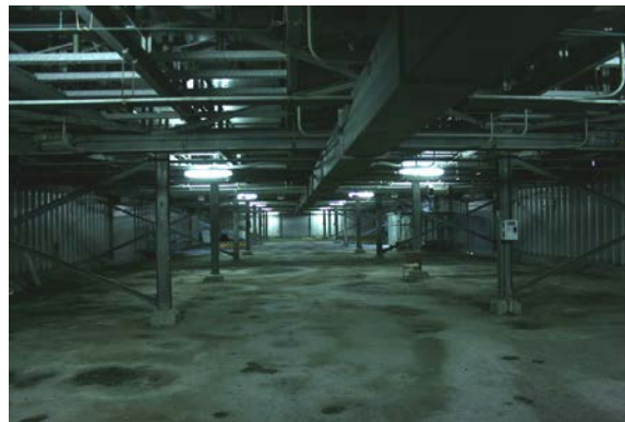
Figure 33. Interior of switchbay in 2012 showing dirt floor, metal walls, and elevated conduits (Site B) (source: Witherspoon 2012)
