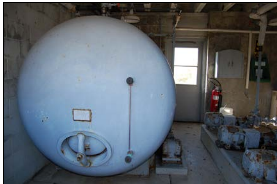
Figure 40. Water tank and, at right, pumps in water storage building (Site A)
