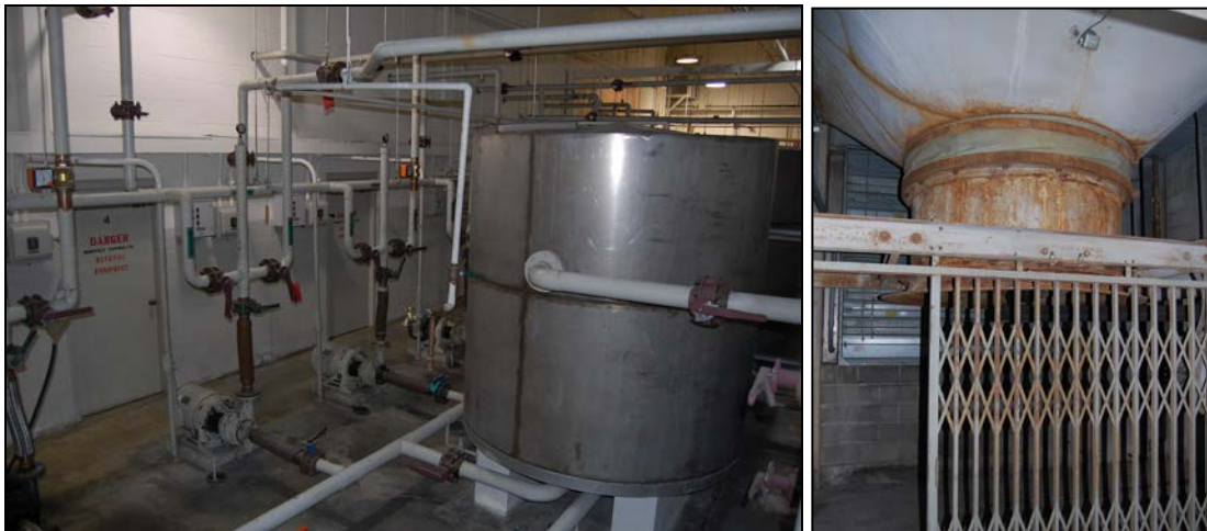
Figure 25. Tank and pump room on north side of building, at left, with doors leading to fan rooms; fan room and fan with louvers at exterior wall, at right (both Site B)
