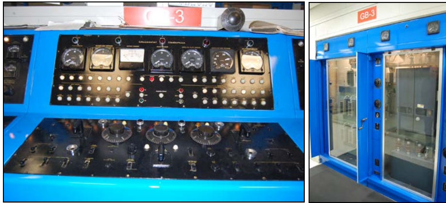
Figure 30. South transmittal hall, console for 250kW transmitter, at left, and the transmitter, at right (both Site B)
