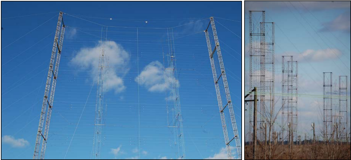
Figure 49. Curtain antenna A-02 with “curtain” of antenna suspended between pair of towers, at left; multiple curtain antennae southeast of antenna A-02, at right
