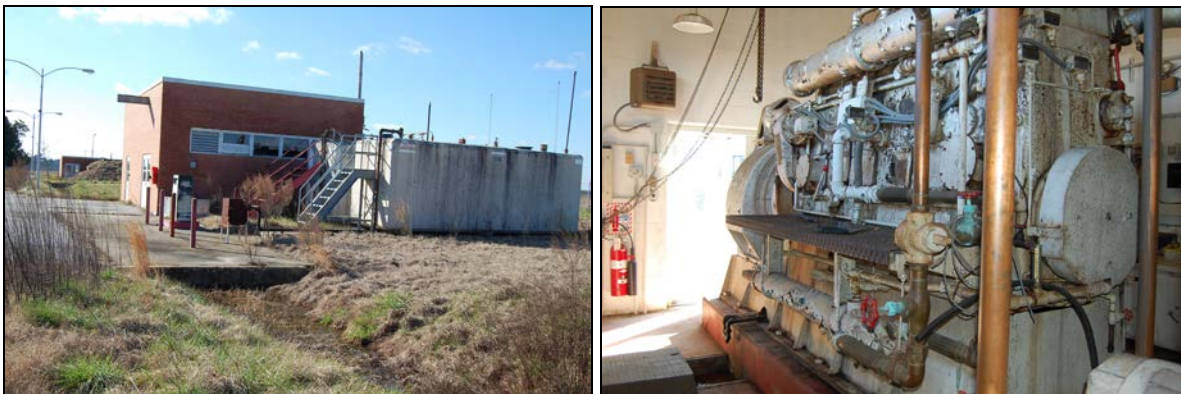
Figure 41. At left, brick generator building and concrete fuel tank; at right, original Chicago Pneumatic Tool Company generator in building
