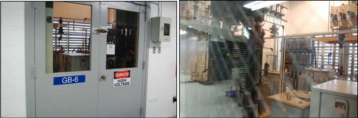
Figure 23. Transformer power vaults along south side of building; note louvered ventilators (Site B)
